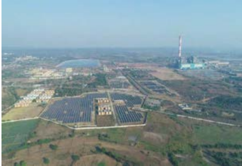
Solar Power Plant at STPP (10 MW)
