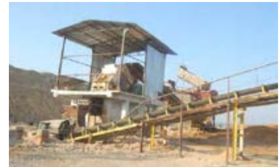
Processed Overburden Plant at Bhupalpalli-KTK OC-II(9 LCM/annum)
