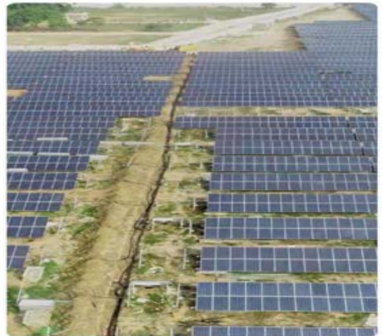
Solar Power Plant at Manuguru (30 MW)
